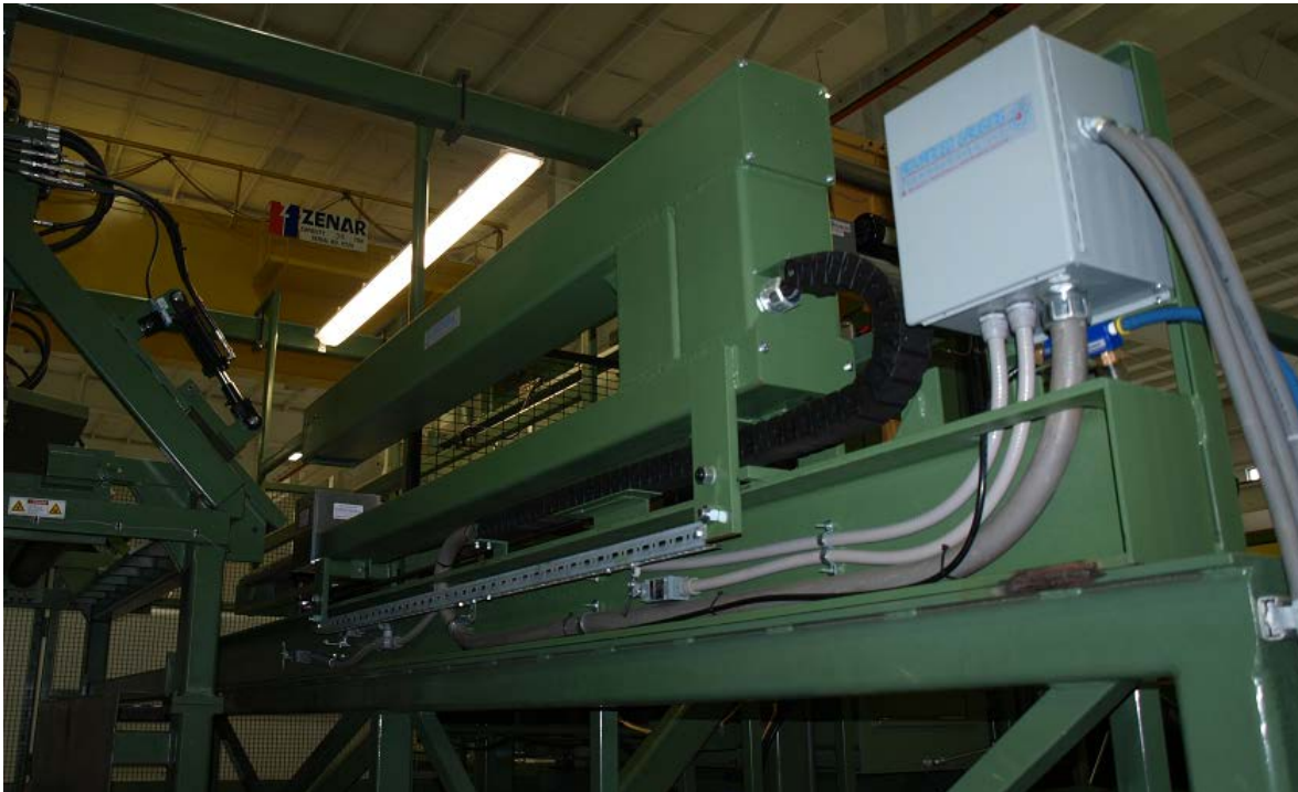
AGT800 Thickness Gauge installed on a 74" EPS Pickle Line AGT800 测厚仪在 74 寸 EPS 酸洗线上的应用
